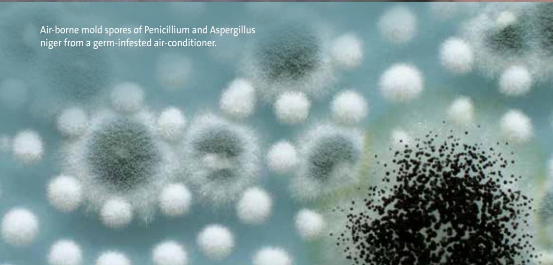
Massive Biofilm Growth (also from an investigated high-pressure humidifier) Apparent biofilm on a pressurized water humidifier that had built-up right into the humidifier basin.
