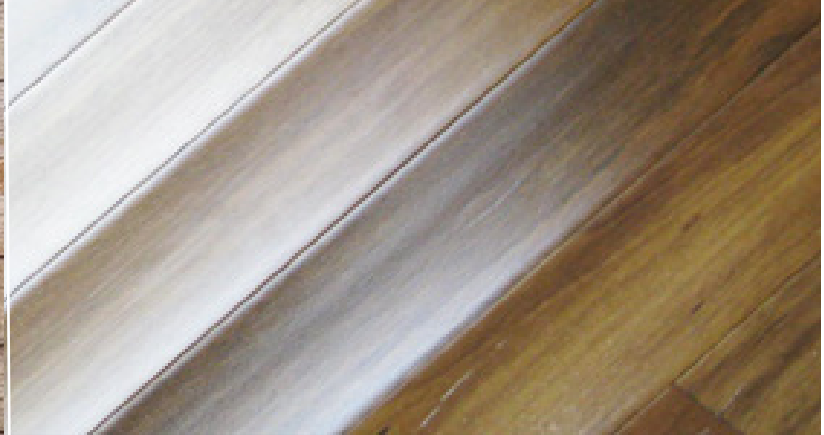
Hardwood floor cupping due to high air humidity levels.
