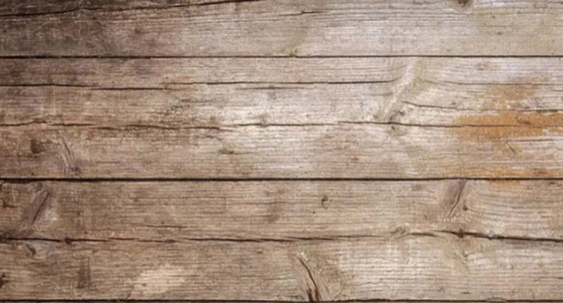
Hardwood floor cracking due to low air humidity levels.
